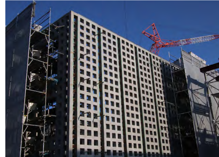
13: Strain gauges were attached to the steel plates and demonstrated that stresses caused by concrete shrinkage would not affect the bearing capacity
